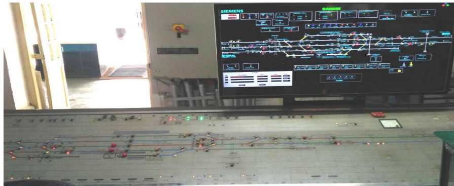
SANCHI STATION OPERATING PANEL AND VDU OF ELECTRONIC INTERLOCKING
