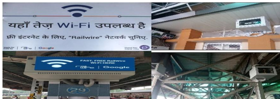
Free Wi-Fi has been commissioned at Saugor station
