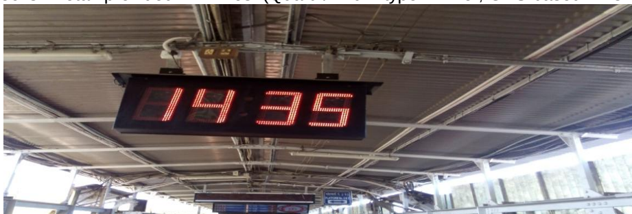
GPS clock at Bina station
