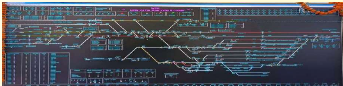
VISUAL DISPLAY UNIT OF OPERATING CONSOLE OF ELECTRONIC INTERLOCKING AT NKJ 'B' STATION OF JABALPUR DIVISION
