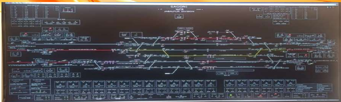
VISUAL DISPLAY UNIT OF OPERATING CONSOLE OF ELECTRONIC INTERLOCKING AT SAGONI STATION OF JABALPUR DIVISION
