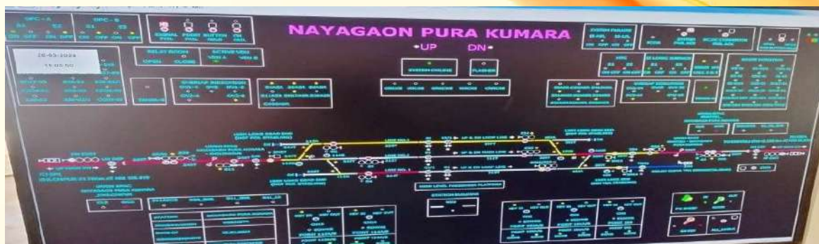
VISUAL DISPLAY UNIT OF OPERATING CONSOLE OF ELECTRONIC INTERLOCKING AT NAYAGAON PURA KUMARA STATION OF KOTA DIVISION
