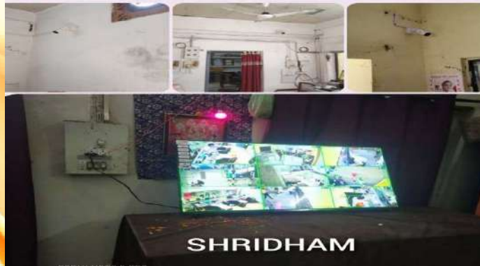
CCTV Cameras (ABSS) at Shridham station
