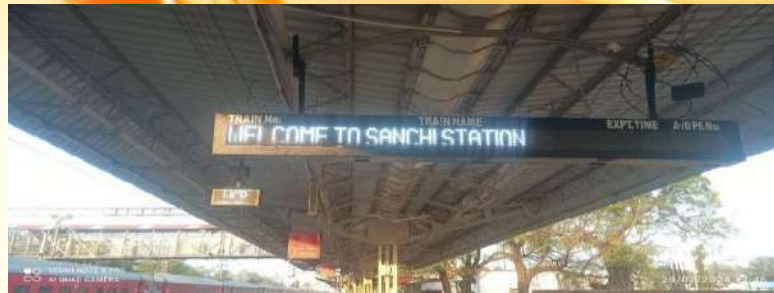
Train Information Display Boards (SLDB) at Sanchi station
